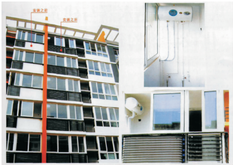
图6 北京清上园小区的住宅太阳能集热系统 Fig. 6 Residential solar heat collecting system, Qingshangyuan Community, Beijing
