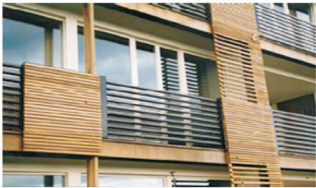
图4 2001年瑞士与建筑阳台一体化的真空管式集热板 Fig.4 Balcony-integrated evacuated-tube collectors at the Sunny Woods, Switzerland in 2001
